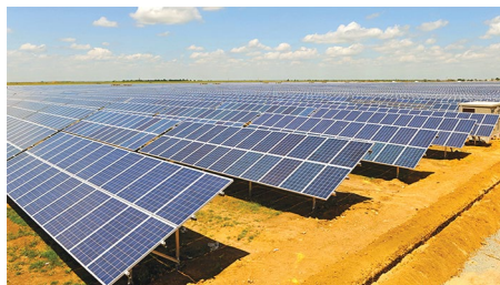
Solar power plant
